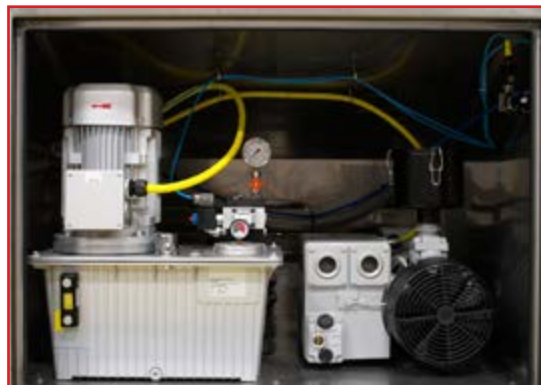
Onboard Hydraulic Power Unit & Vacuum Pump Motor
